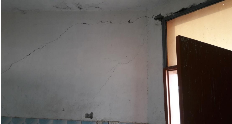
Cracks on the Walls on the inner side of the Room
