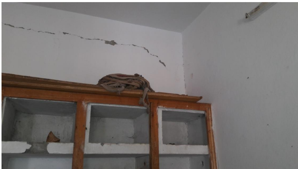
A Prominent Crack on the Walls on the inner side of the Room
